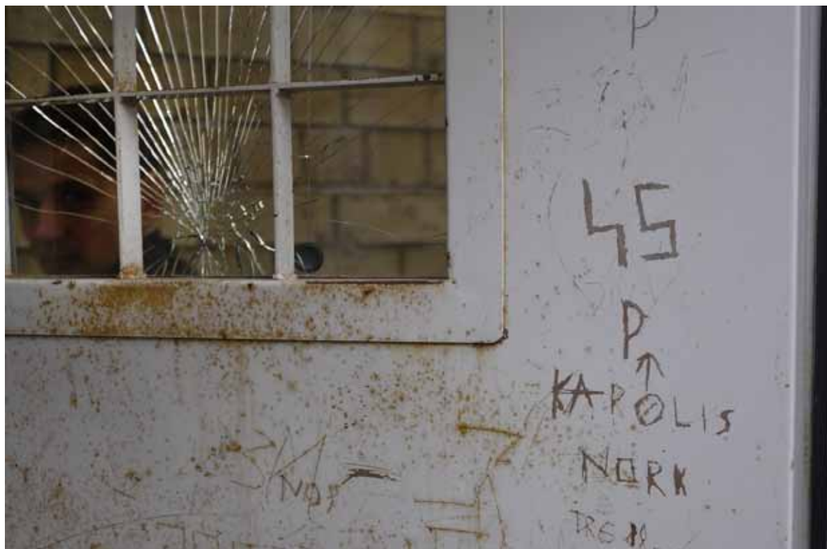
Fig. 3. Internal door of isolation unit
